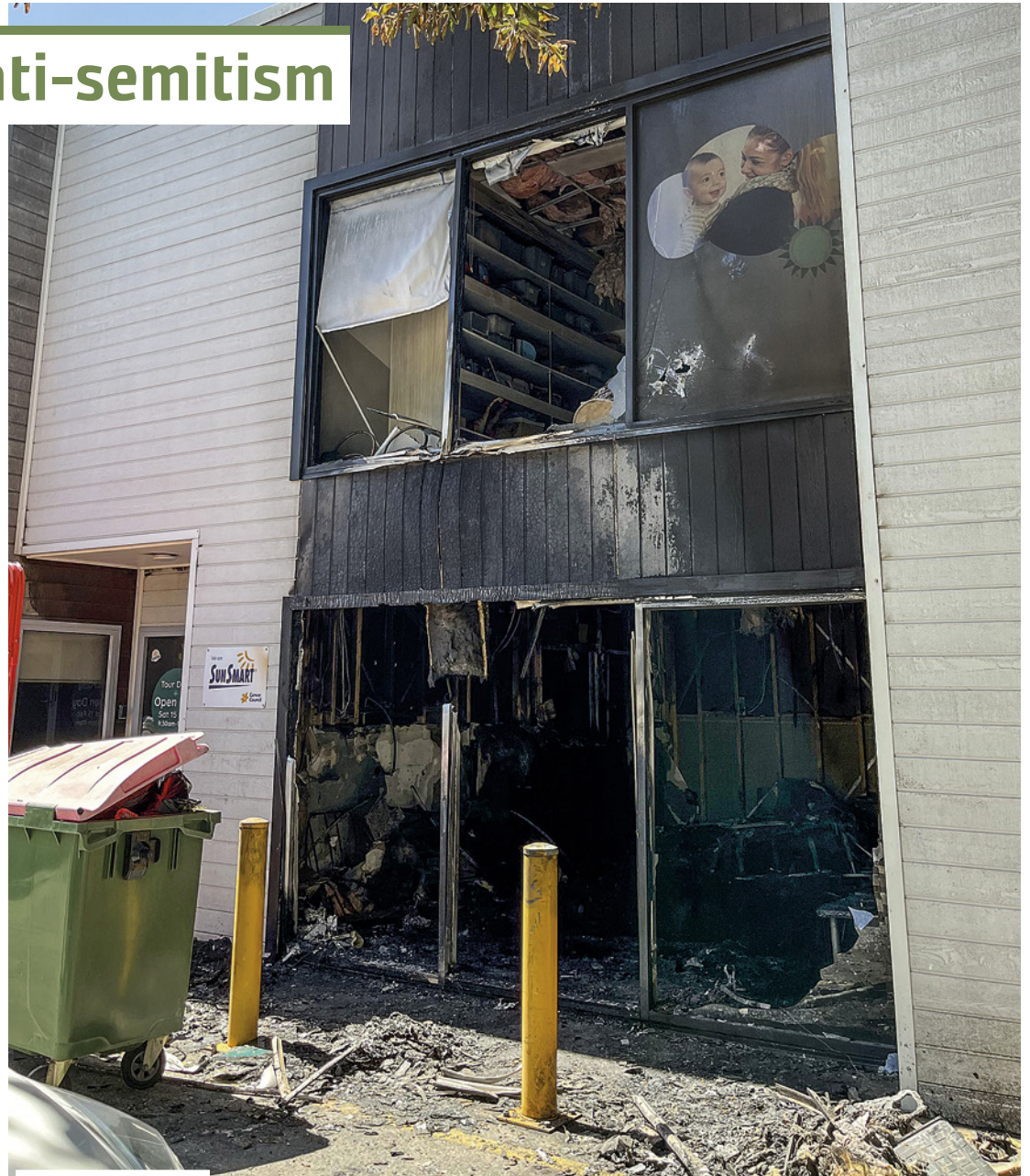
Yet another attack: fire damage at the Only About Children centre in Maroubra.
